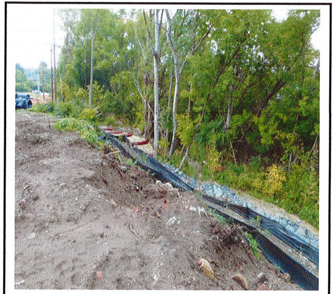
Area where water is coming onto the site. Consultant has developed a plan to address this.
