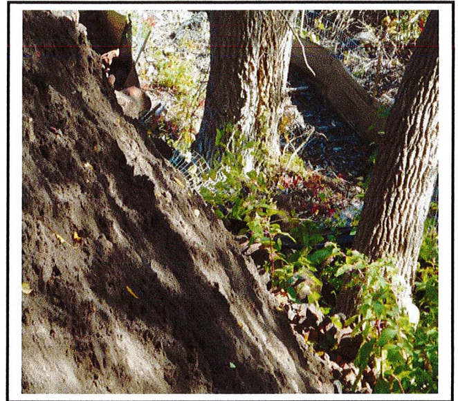
Silt fence located by construction trailer, requires replacement. Fill has been pushed on top of it.
