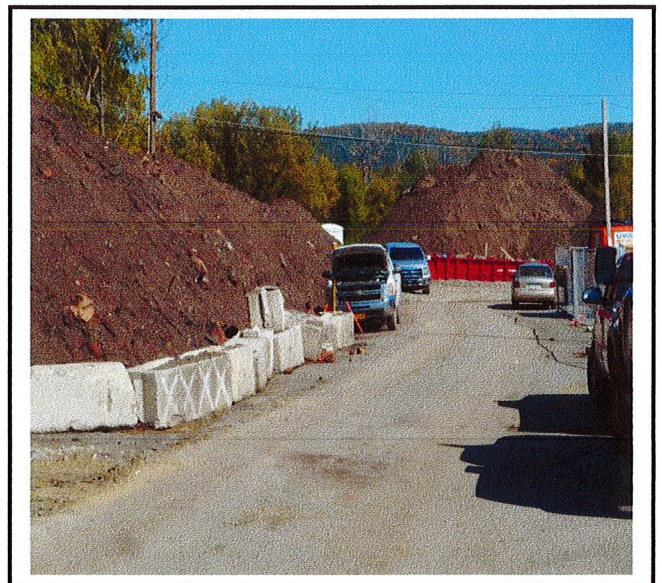
Stockpiles that have sat idle require stabilization.
