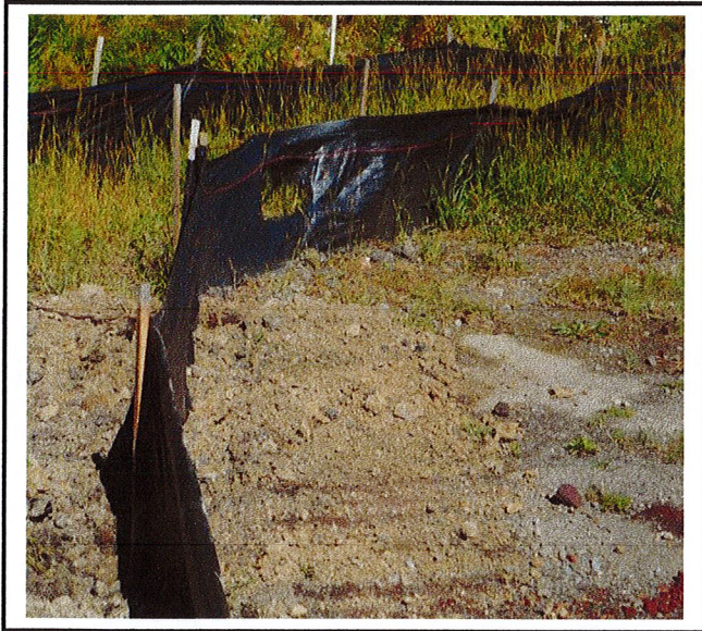
Silt fence located on the North east end of the project requires repair.
