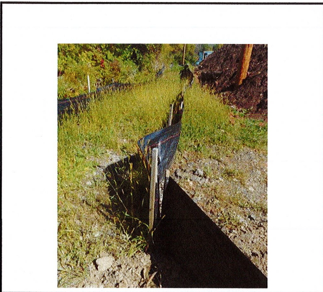
Silt fence along Northeast end of project the splice does not meet standard.
