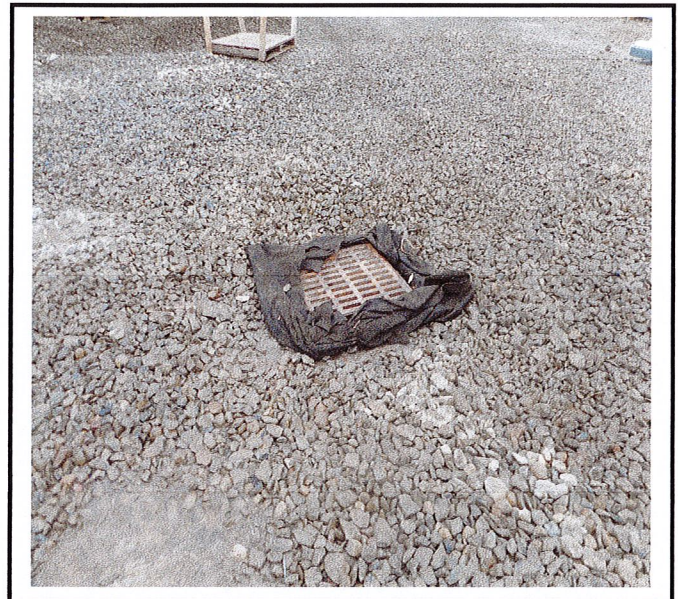
Drop inlet protection requires immediate repair.
