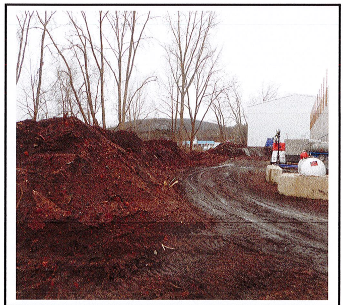
All stockpiles require stabilization.
