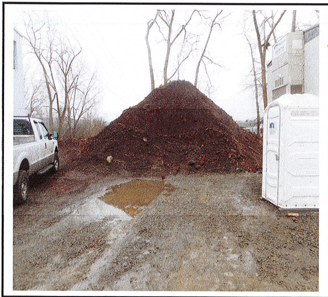
All stockpiles require stabilization.
