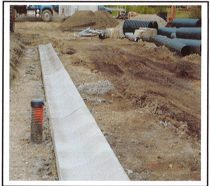
Excess concrete disposed of improperly.
