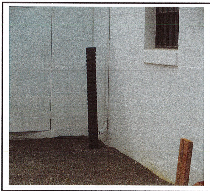
Roof drain (on existing building) not connected to system.
