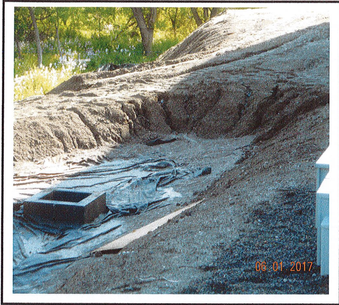
Bioretention area has not been completed. Bare soil has been left open and is now eroding. This silt will need to be removed and stabilization is required.
