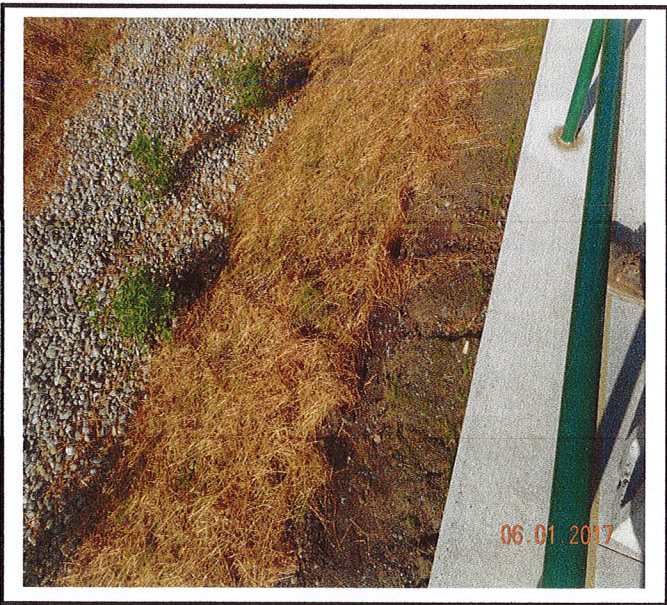
Side slopes of bioretention #2 require further erosion control efforts.
