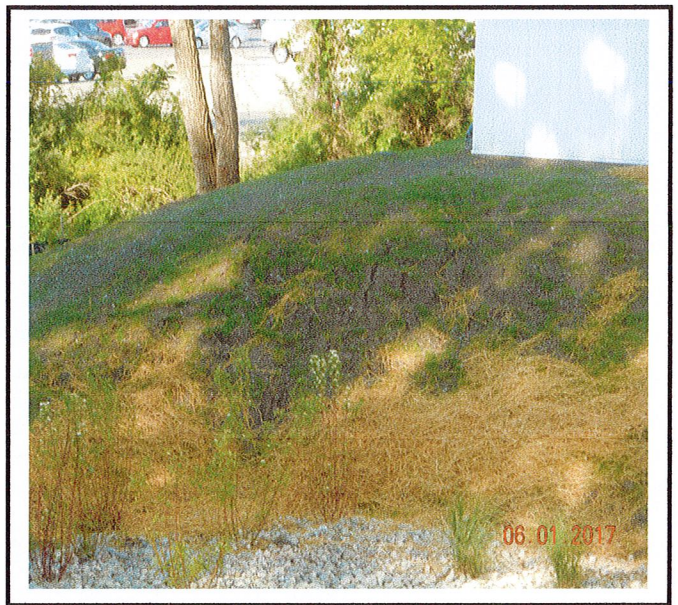
Further erosion control efforts are needed on these slopes.
