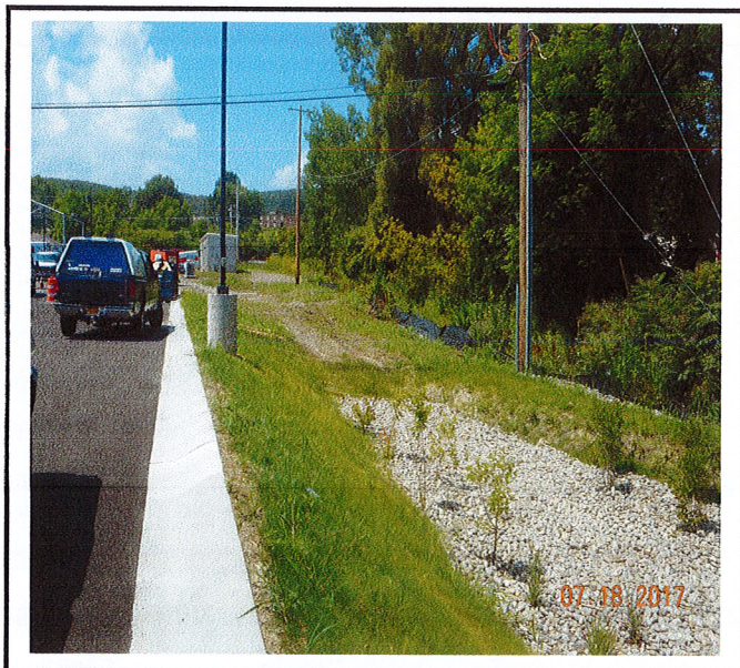
Slight erosion and sedimentation is creeping towards the bioretention from unfinished basin.
