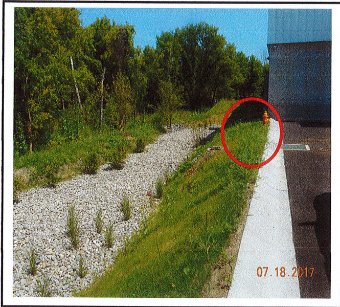
Rock slope protection has not been installed.
