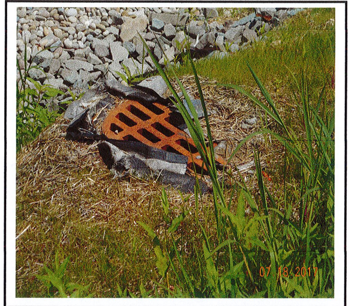
Silt Sack will need to be removed from this structure.
