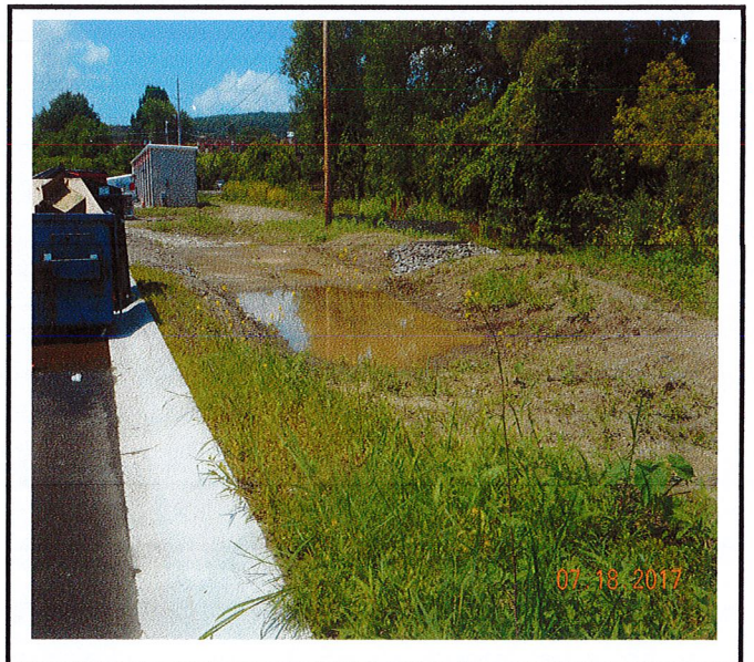
Unfinished stormwater basin. Erosion is occurring off the back of building b into the basin.
